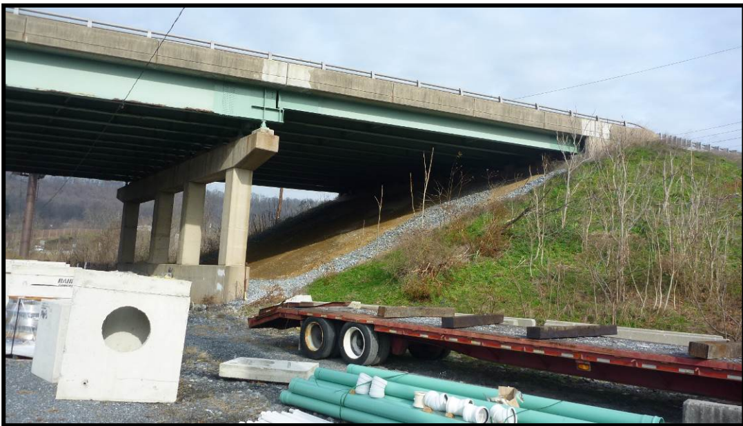
Photo 12: Eastern span of the bridge looking at pier 2. Option A proposes to build trail behind the pier.
