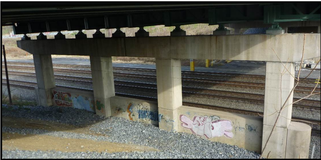
Photo 14: Rear face of the western pier to be used to connect to Fort Hunter.
